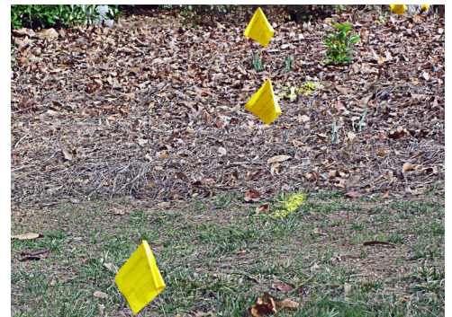
Markings help identify the locations of existing utilities in a project area.
