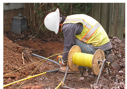
Connecting the service line to the main line usually happens in the right-of-way but may require some work on private property.
