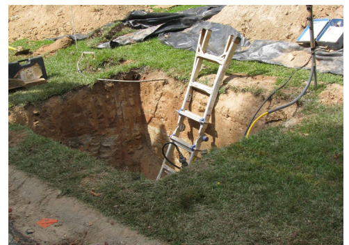
Crews dig areas like this one when installing pipe via the directional drilling method.
