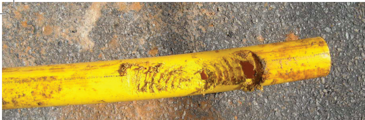
Natural gas piping damaged during cleaning operations
