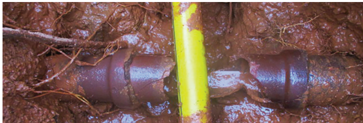
A sewer line penetrated by natural gas piping
